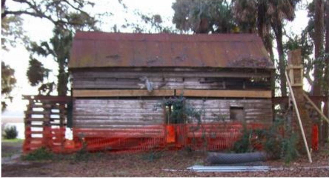
Figure 3.3 Garvin House Stabilization This image shows the Garvin House after initial stabilization, c. 2008. Image courtesy of Erin Schumacher
