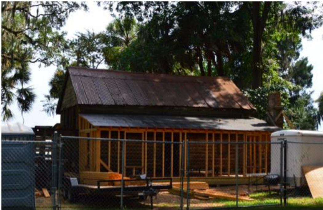
Figure 3.6 Rear Lean-to Reconstruction This image shows the reconstruction of the Garvin House rear lean-to, c. 2016. Image courtesy of Erin Schumacher
